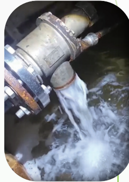
Abnormal conditions occurred in saltwater supply system 鹹水供應系統出現異常狀況
