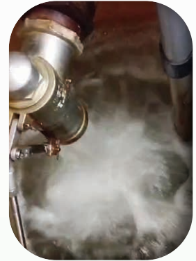
Normal condition of saltwater supply system after repair 鹹水供應系統修復後正常狀況
